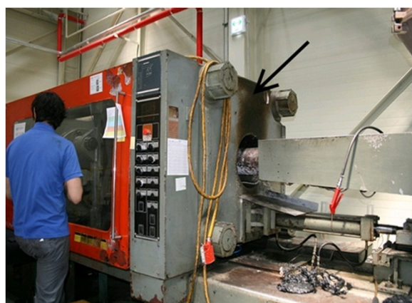
Figure 2 Injection port of the plastic resins (pouring resins into the hopper of the molding machine). The arrow indicates discoloration caused by hume leakage when injection processing or changing the raw material.
